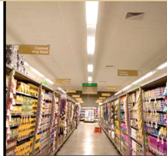
Rouse Hill has automated lighting control.
